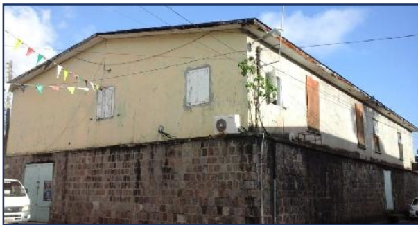
Pic A - the Cotton Ginnery House. A facility, which once housed the Department of Culture and the Nevis Sports Museum.
