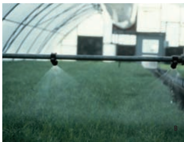
Figure 10.16 —(A) Moveable boom irrigation systems (B) apply water in a very efficient linear pattern but may be considered too expensive for many small native plant nurseries. Photos by Thomas D. Landis
