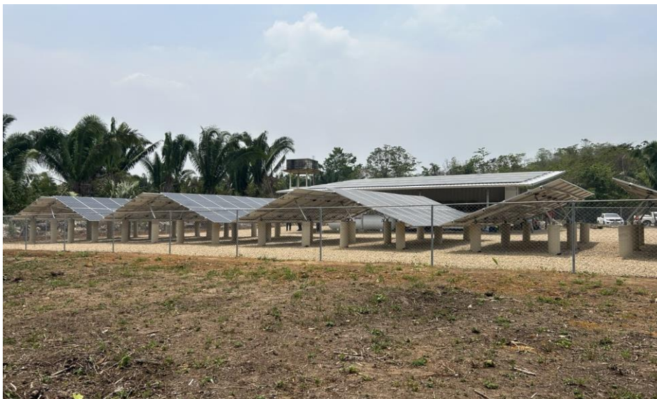
Figure 17: Front Elevation of the entire power generation unit.
